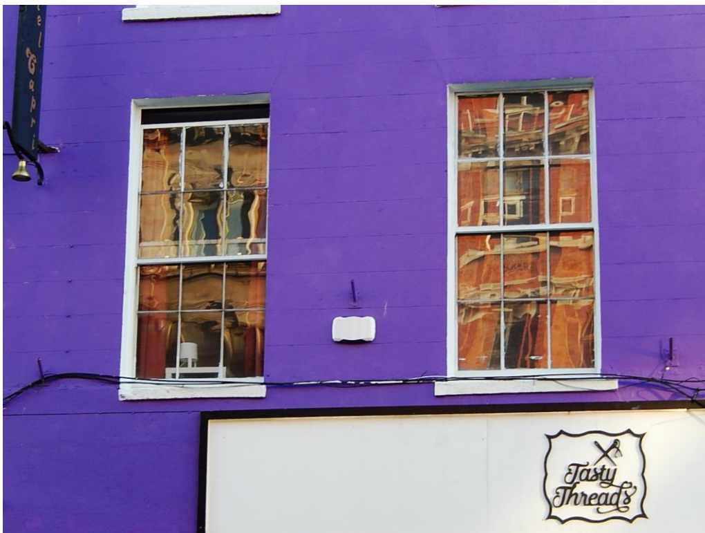
First floor windows at 58 Abbey Street Middle showing historic glass still intact.
